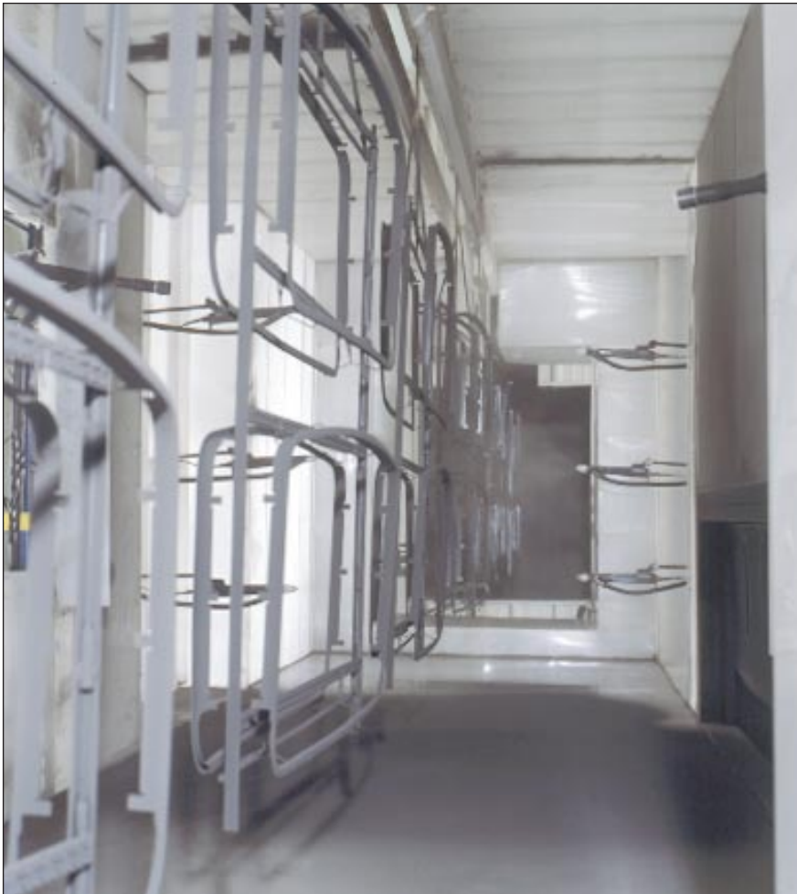
Automatic corona-charging guns apply powder coatings to parts. The system automatically recycles and reuses all powder that does not go onto the parts, boosting overall efficiency.
